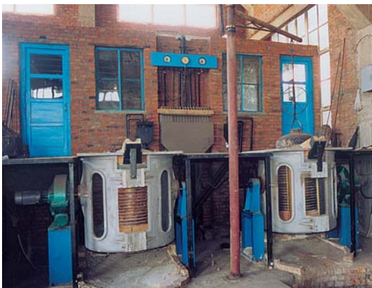
MIDDLE FREQUENCY FURNACE
